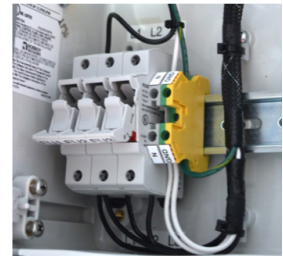
Fused voltage terminations
