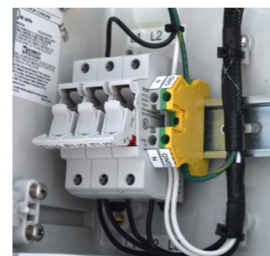
Fused voltage terminations
