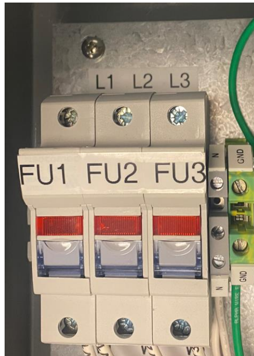
Figure 3: Wire the voltage based on the labeled fuse holders (note that the fuse holders are empty).
