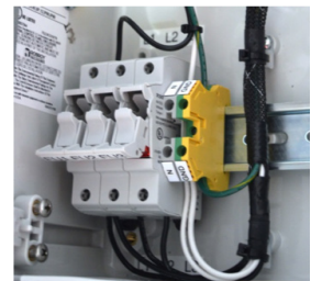
Fused voltage terminations
