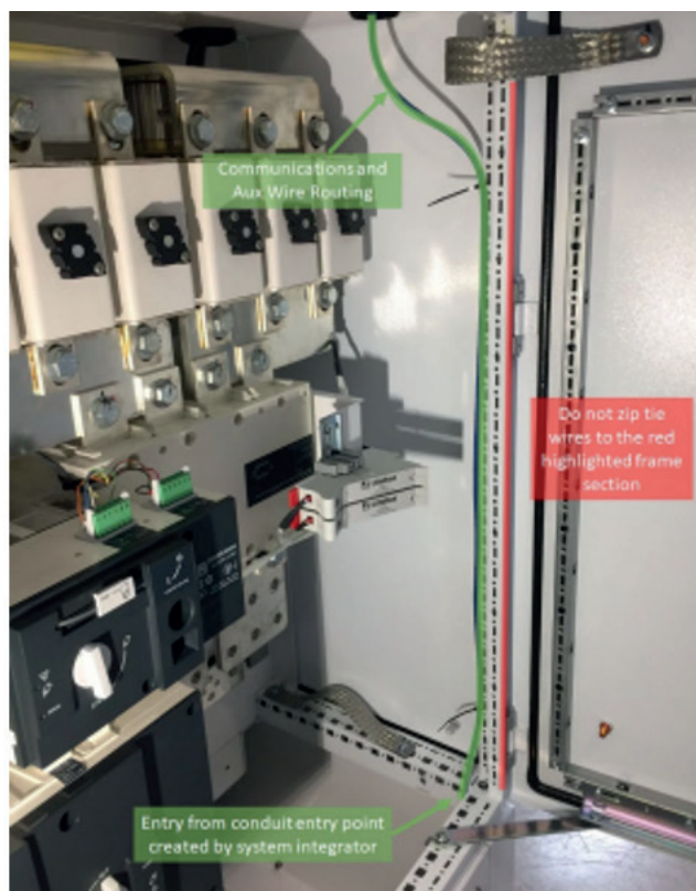
Figure 124. C-Cab XXL Lower Cabinet Auxiliary and Communication wire routing to the User Interface
