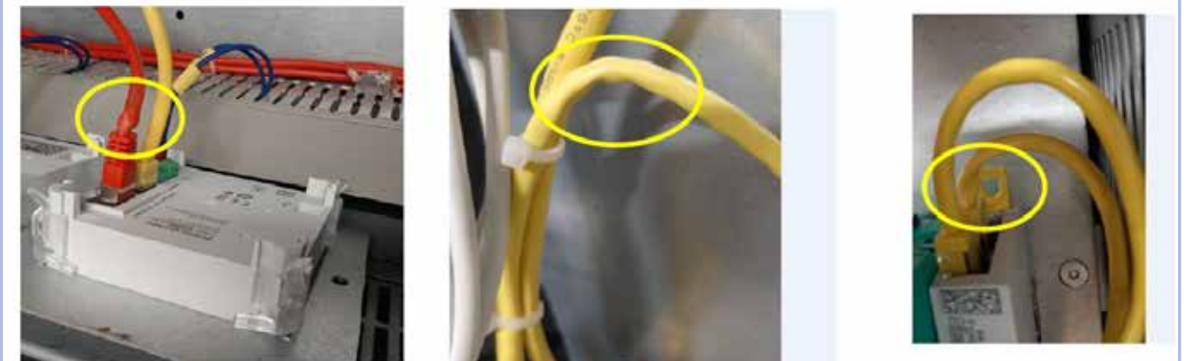
Fig. 13: Examples of poor RJ45 cabling.
