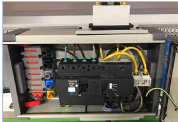
Fig. 10: Socomec withdrawable connector tap off box integration.
